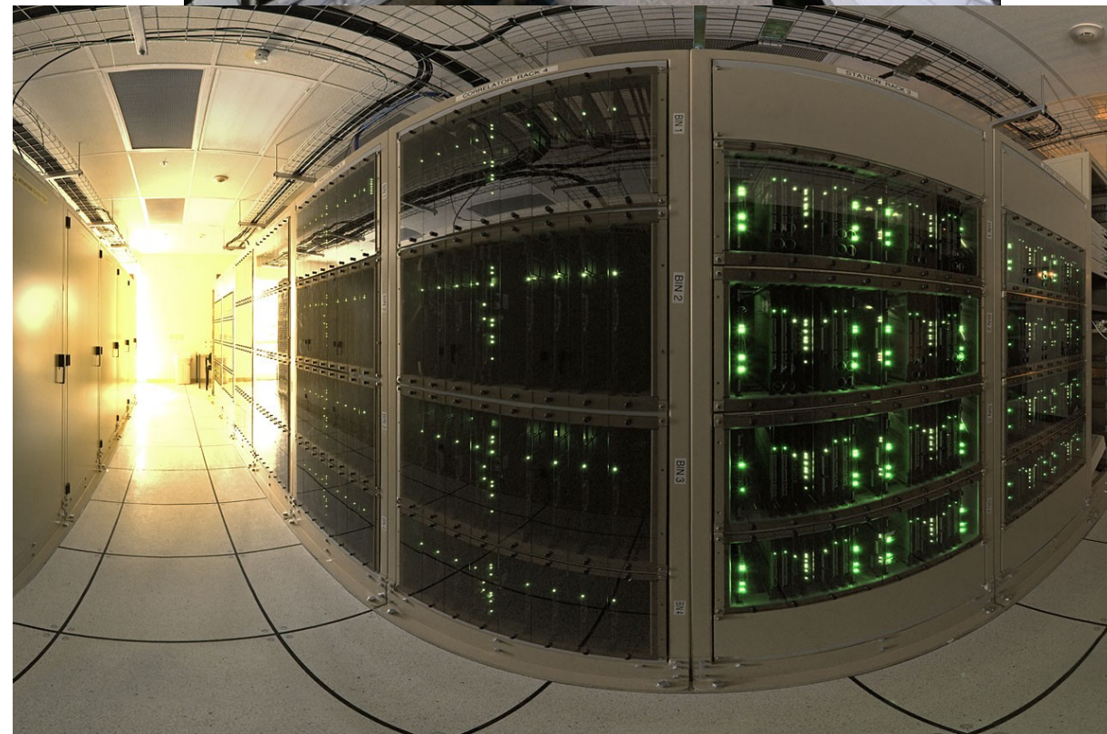
ALMA correlator with over 134 million CPUs. It performs up to 17 quadrillion operations per second, a speed comparable to the fastest general-purpose supercomputer in operation today.
