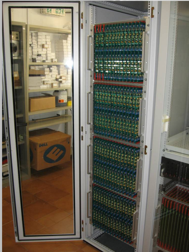
Filter bank rack
